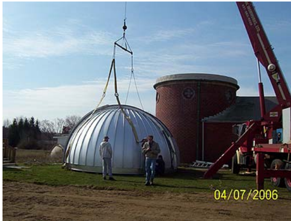
A view southwest as the sling is affixed in preparation for hoisting
