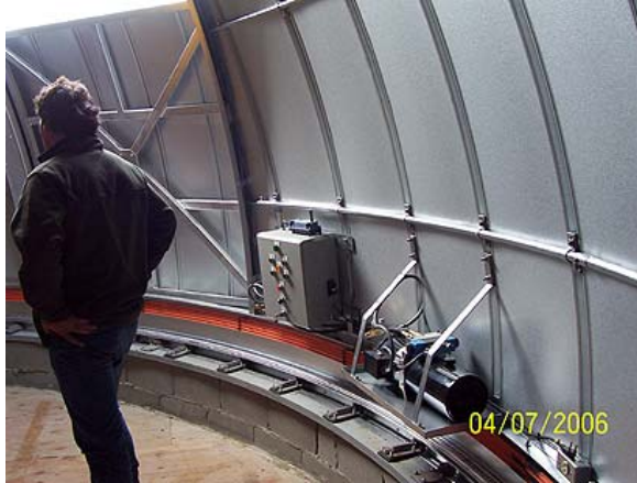
Kurt takes a break and ponders the many new challenges as they present themselves. The electro-hydraulic controls are to his right.
