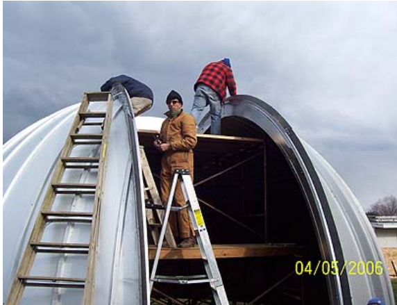
David assists in the final assembly and adjustment of the shutter track. The shutter consists of 3 sections, 2 joined together at the top that slide along the track with the 3 rd , hinged at the base, that opens out.
