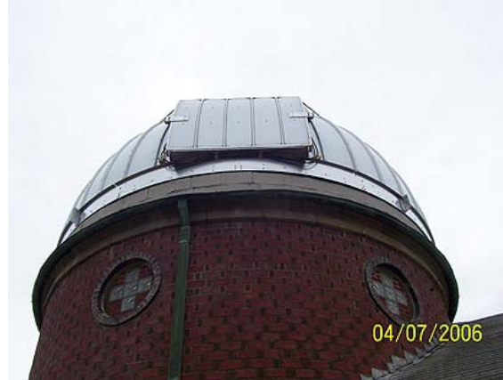
The fully-secured dome stands ready for the next step, the installation of our new, observatory-class telescope.
