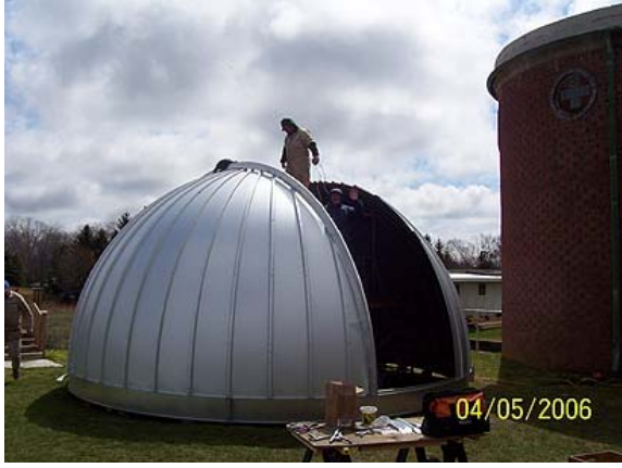
Brian stands atop the scaffolding necessary to access and assemble the shutter track and dome crown section. Rich is to his left.
