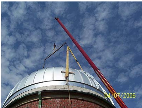
Having been just placed atop building, the new dome waits to be secured in place
