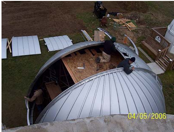
As the dome takes shape, a bird's eye view of the hardworking crew from what will be its permanent perch.
