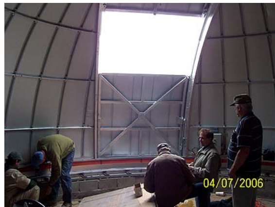
Everyone works hard as the dome is permanently secured to the base rim
